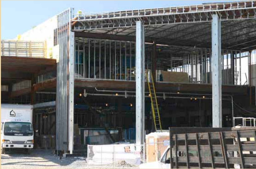
Construction to expand the SMC has required the relocation of most offices and activities over the summer. The University Store remains open.
